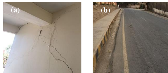
Fig. 1: Damaged structures in Kohat Cantt (a) Building and (b) Road
