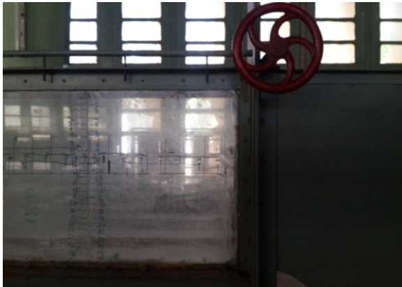
Fig. 2. D/S gate opening/ closing wheel mechanism
