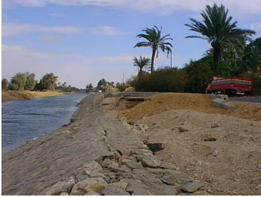
Figure 4 : Slope failure of case 1
