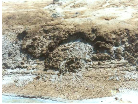
Figure 5 : Salt leaching and slope failure of case 2
